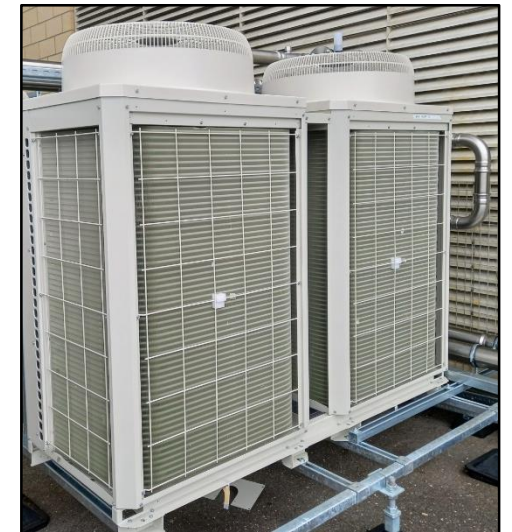
Heat pumps at Exe Valley Leisure Centre
